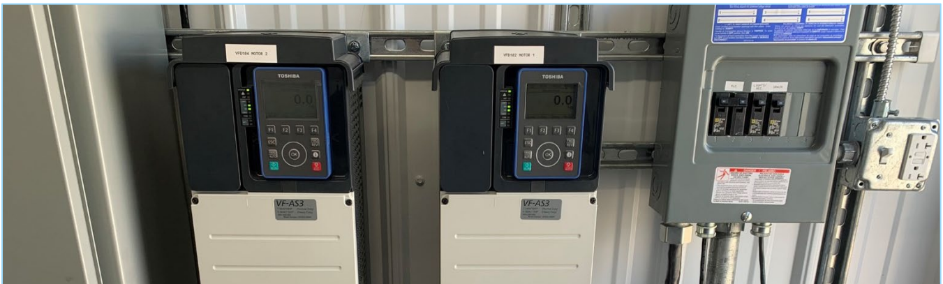
Motor drives regulate the compressor speed to match the air needs of the pad.
